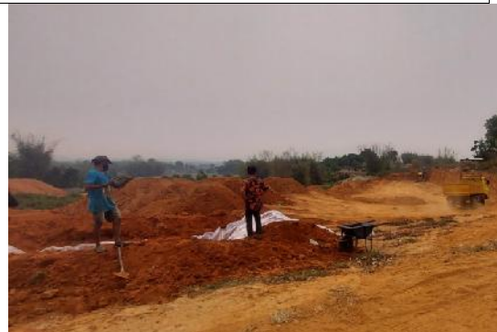
Proposed Dudhauri Substation Location
