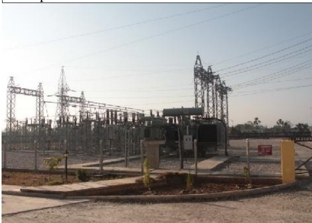
Hardi Substation. It is the tapping point
